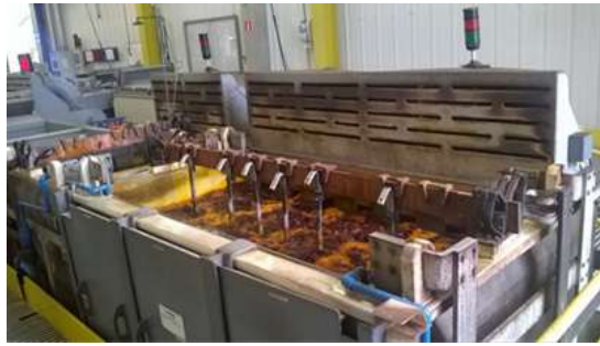
Figure 3: Fixing devices fitted into the busbar of the chromic anodizing tank
